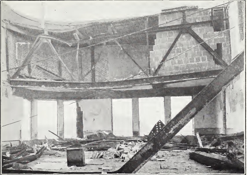
A. ROOF TRUSSES DAMAGED BY HEAT, THROUGH FAILURE OF TERRA-COTTA COVERING, MUTUAL LIFE BUILDING, SAN FRANCISCO.
